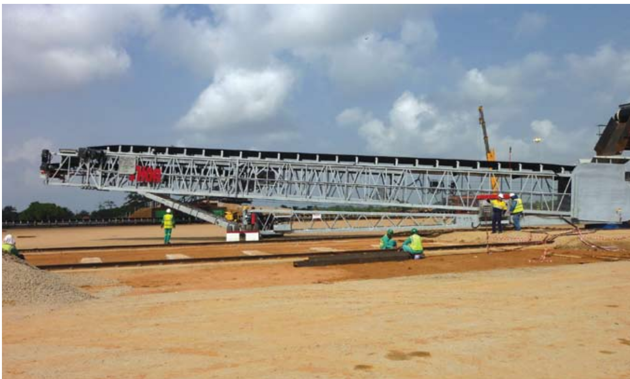
Setting up of the telescopic stacker at Pepel Port for dry commissioning.
