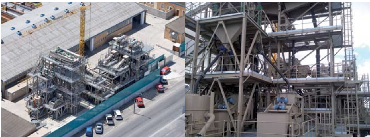
EPE modular plant.
