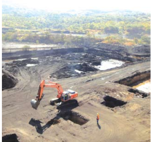
Progress on site for a modular coal handling process plant, with ROM feed of 2.4 mtpa and washing plant process capacity of 200 tph, for Maamba Collieries Ltd in Zambia.
