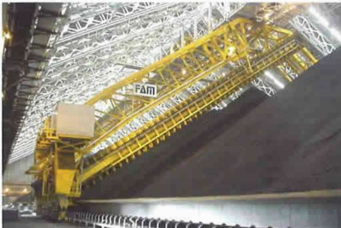
Portal scraper re-claimer in covered stockpile, with a gauge of 69m and a throughput of 2 000tph – installed in Taiwan.
